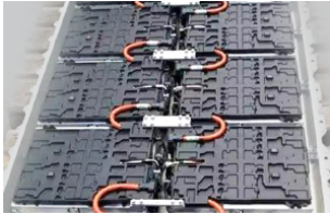
Battery charge/discharge test
